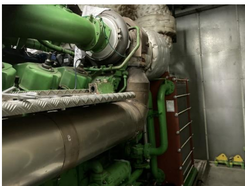
Part of a CHP unit
