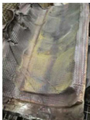
Yellow dust deposits beneath section of insulation
